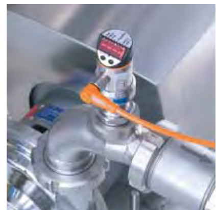
A bar graph displays the state of the pump on the unit.
