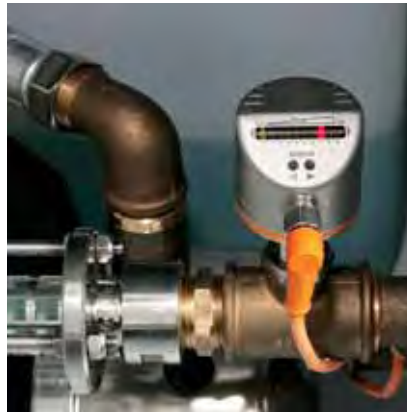
Use of flow monitors for monitoring seal water on pumps.
